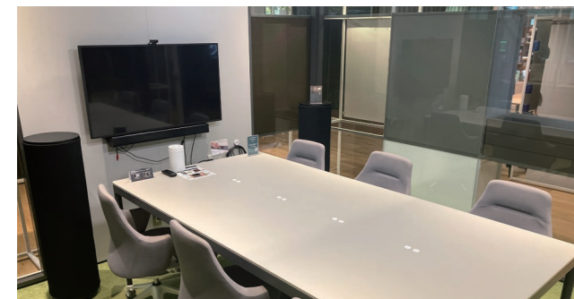
Installation of a product that suppresses reverberating sound in a meeting room
