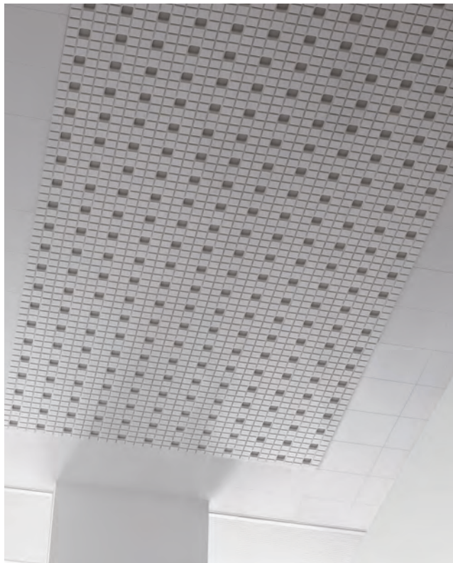
Ceiling Material: Acoustic Ceiling Panel (Modern) AcousticBlock TB0210 Acoustic Ceiling Panel (Modern) 15 TB0213
